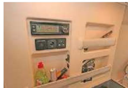
It looks like a radio but it controls the fridge, heating and hot water
